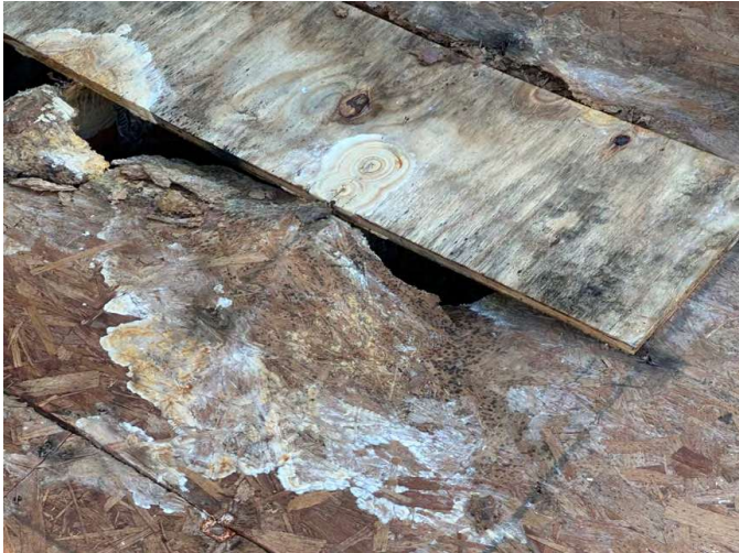
Photo 5: Rotten wood - moisture-damaged OSB which is the result of condensation within and above the OSB Board.
