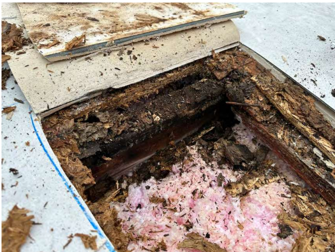
Photo 6: Deteriorated Roof Structure - concern with heavy, wet snow.
