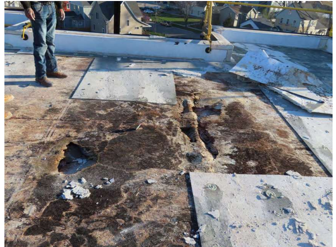
Photo 11: Scary Roof Deck Conditions! Who gets to pay for corrective work?
