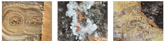
Photos 8-10: Severe mold growth on OSB underside.
